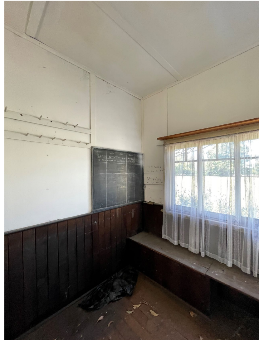
Figure 41: Croquet Equipment Store original windows
